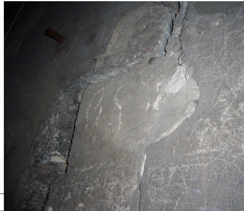
Partially filled segment of a crack
